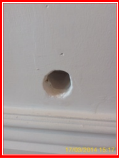
4.3.3 Two holes between windows and electric fire.
