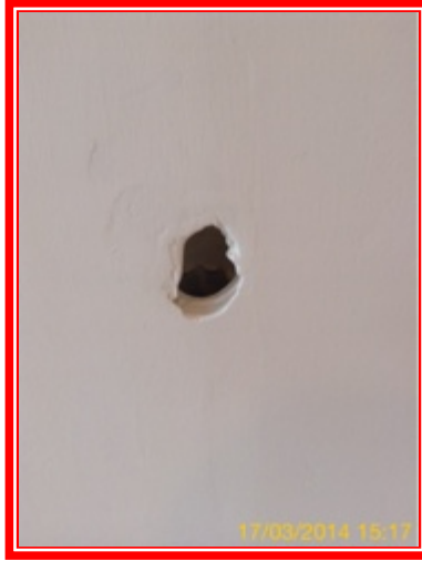
4.3.3 Two holes between windows and electric fire.
