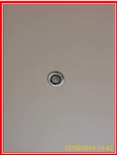
4.5.1 1 x Recessed Spotlights bulb(s) not working.
