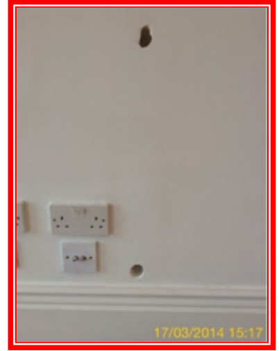
4.3.3 Two holes between windows and electric fire.
